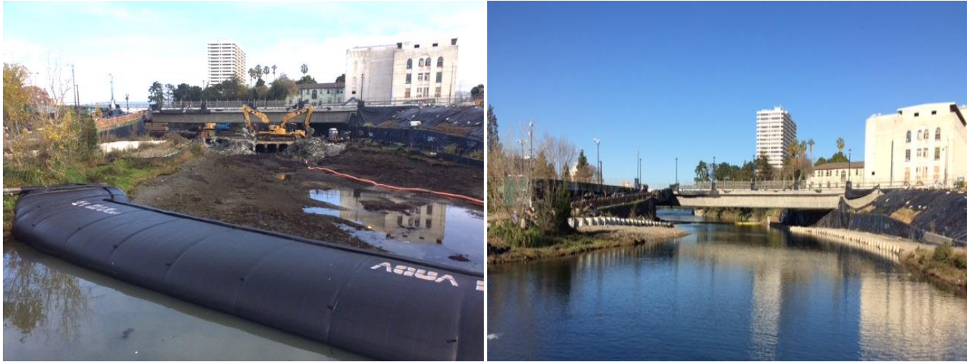
(Photos: Joel Peter; Oakland Public Works, Retired; January 2016; Project underway and near completion)
